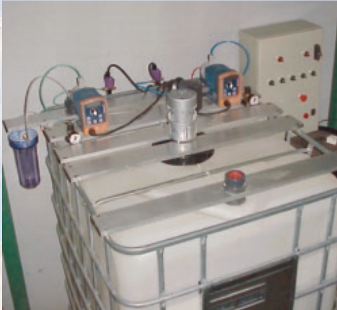
Feeding power station
